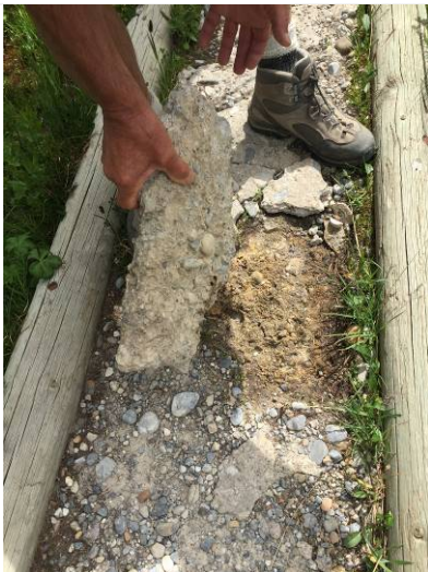
Concrete failure on Opabin Plateau
