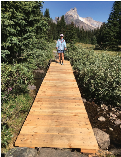
Morning Glory Trail at Elizabeth Parker Hut: Installed a new bridge over the creek from which hut guests retrieve water. Photo: Sue Webb.
