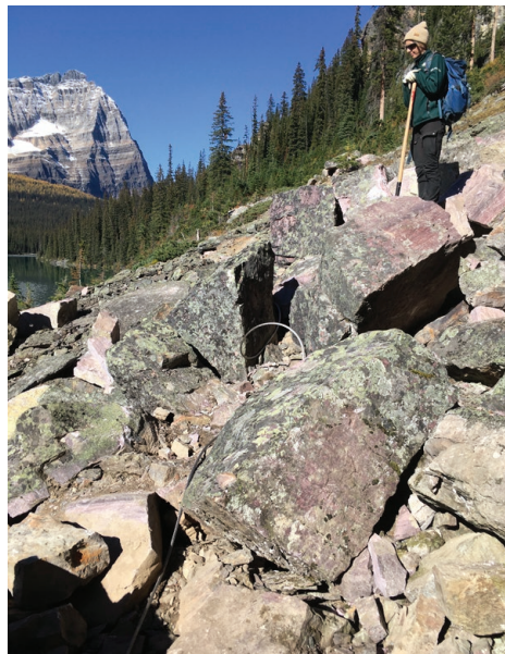
In September 2023, a large rockslide consisting of refrigerator-sized boulders swept over the south end of the Lakeshore Trail. Repair work will continue into 2024.
