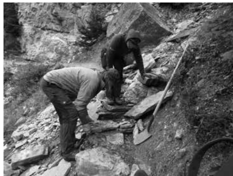
Trail crew members Steve Bertello and Lauren Goforth repair damage from avalanches on Lakeshore Trail. Photo: Sue Webb
