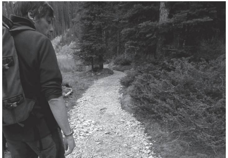
Lakeshore trail flood damage repairs. Photo Judy Otton
