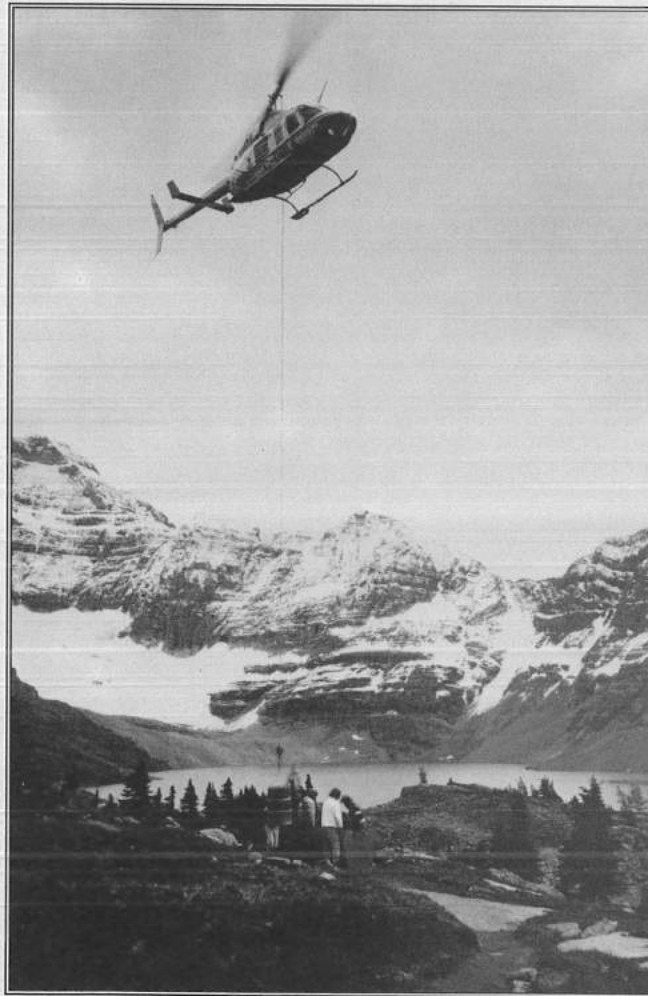
Helicopter transported gravel is used to resurface the Lake McArthur Trail Photo courtesy of Don Gardner
