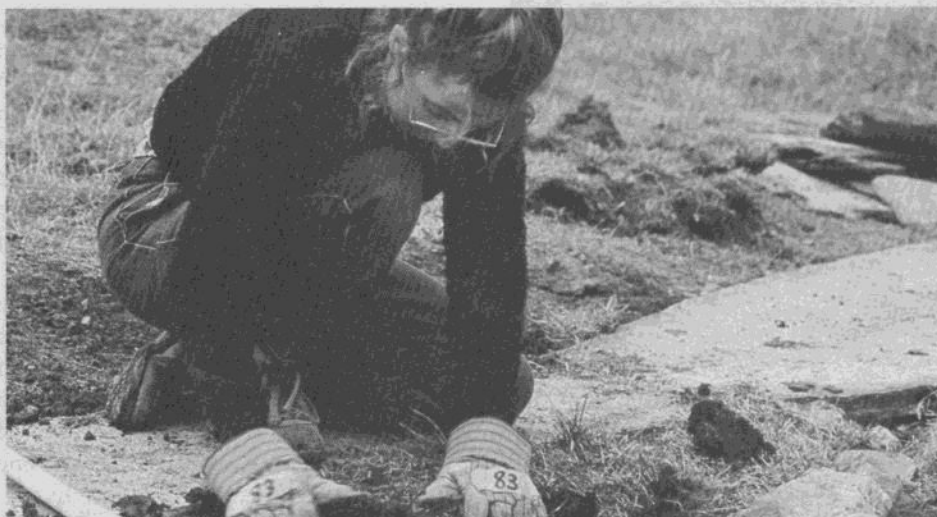
Diny Harrison fitting large slabs to provide a solid, stable walking surface.
